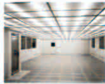
Modular Cleanrooms – Vertical Flow HARDWALL
