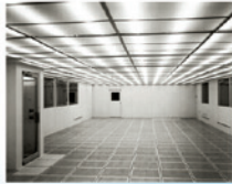
Modular Cleanrooms — Vertical Flow HARDWALL
